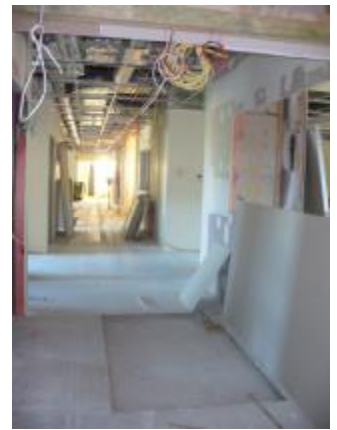
The History corridor has been replaced with a new corridor located within the new ICU. The indent in the floor will be a bed weighing station.
