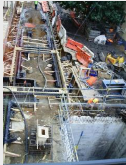
Straight ahead is the link from the AMC to Edmund Hillary Block. On the right is the new lift shaft
